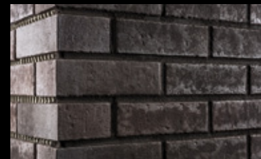
The finished joint pattern. Full masonry stretches are grouted at one go.
