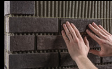
Use a string to plumb the clinker area. The clinker slips are pressed into the adhesive bed.
